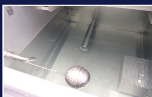
STEAM MIXER & FLOAT SWITCH
